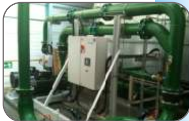
Air Conditioning Plant
