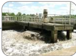
Effluent Treatment Plant
